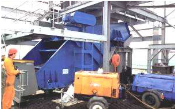
Multi angle screen installed in a coal washery
