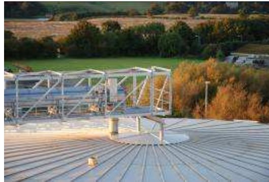
View of feed to 350 te GKV vessel.
