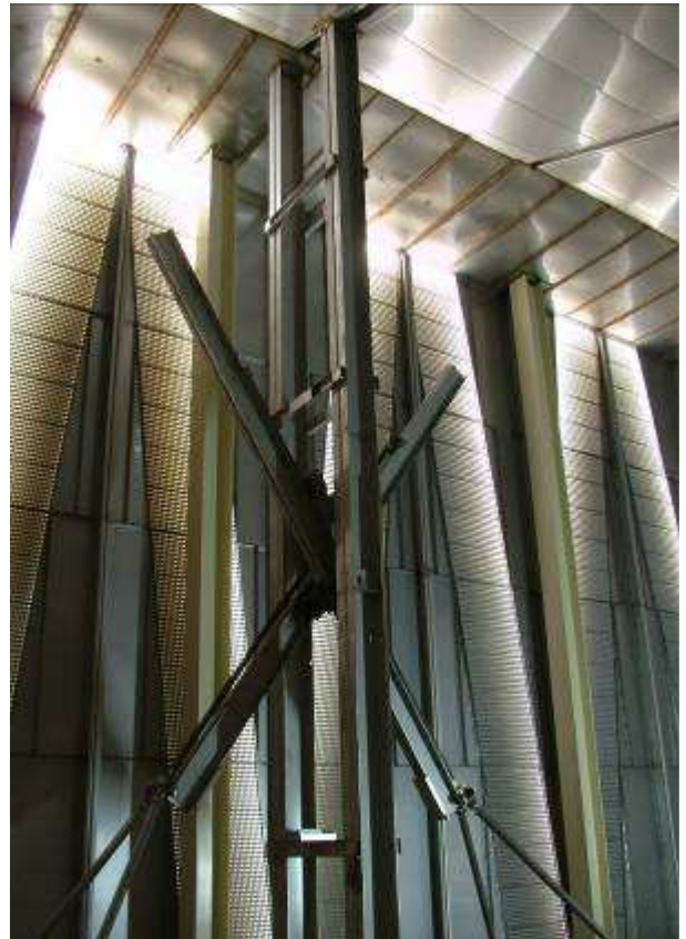
Recirculation door operating mechanism inside air intake chamber.
