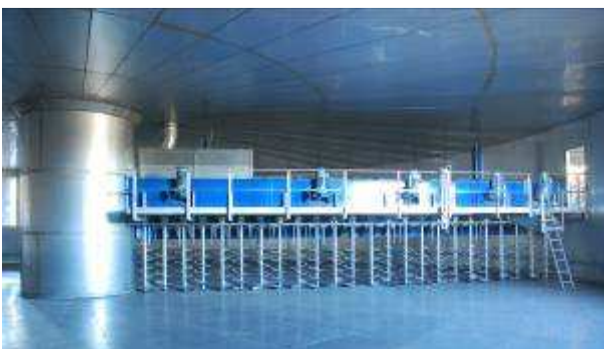
Stripper loader turner in a 30m diameter rotating floor Germination / Kilning vessel.
