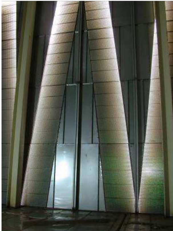
Internal view of air intake chamber showing glass tube heat exchanger for a 20MW (350t batch) kiln heating system. The design gives 80% heat recovery from 1.3t/h of saturated air.
