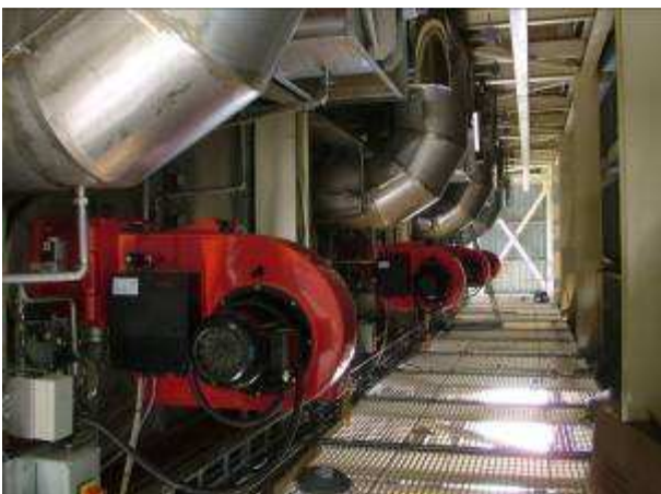
Four 5 MW gas burners.
