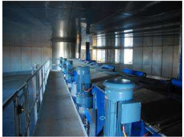
Stripper / loader / turner access walkway.
