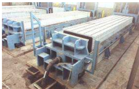
Filter Press House. Used for waste water clarification and the separation of Washery Tailings
