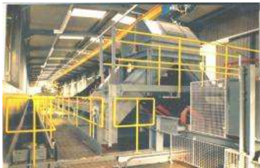
2000 Tonne Capacity Rapid Loading Bunker Tripper Loading Conveyor
