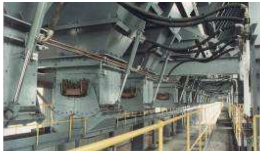
2000 Tonne Capacity Rapid Loading Bunker Hydraulically Operated Clamshell Doors
